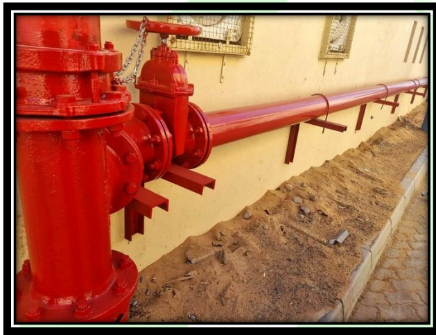
Fire Fighting Line Connection (HDPE/GI) – Bawadi Mall, Dominos.
