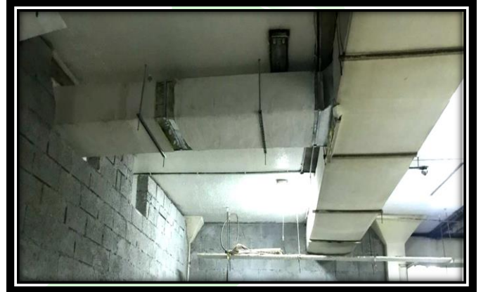
Modern Bakery – MEP Works
