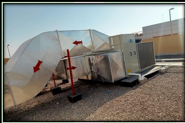
Package Unit installation with Air Duct
