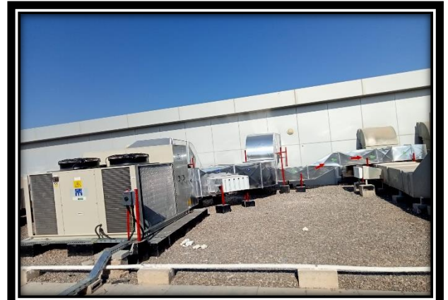
Package Unit installation with Air Duct
